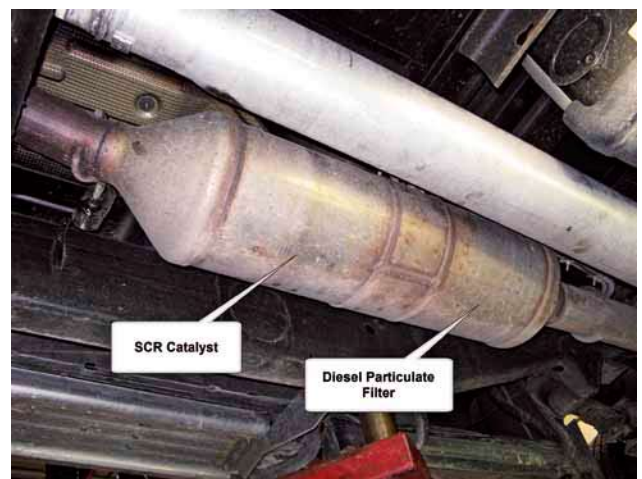
The 2011 Duramax diesel uses an SCR catalyst with a diesel particulate filter (DPF). In this application, the DPF is located downstream from the SCR catalyst.
